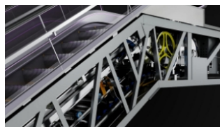
Main drive speed monitoring
